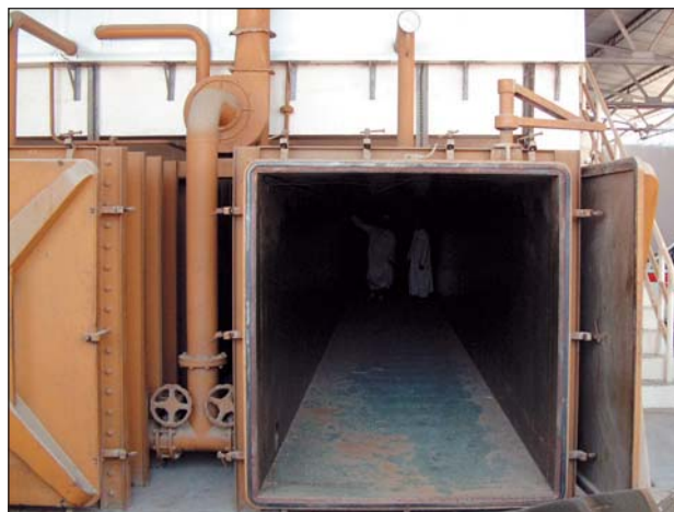
Fig. 2.23. Fumigation vacuum chamber in Sultan Qaboos Port in Muscat, Oman.
